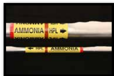
AMMONIA REFRIGERATION MARKERS PAGES 33-34
